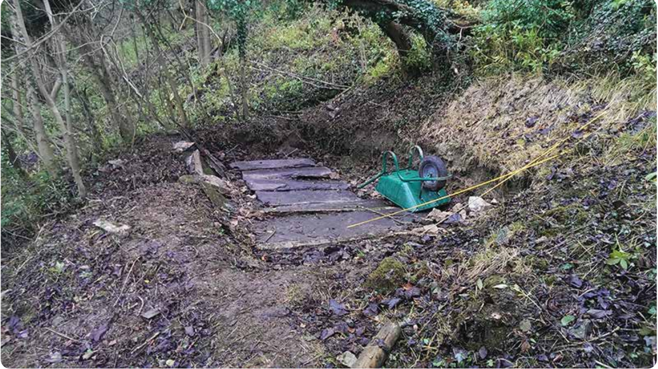
Old heavy slate covers posed a lifting hazard when access was required
