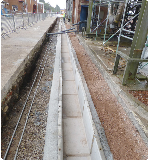
From an initial website search for lightweight composite panels to the installation of 190 new Fibrelite covers
