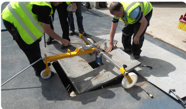
Manual handling: The previously installed damaged cover required a hydraulic lifter to remove the cover
