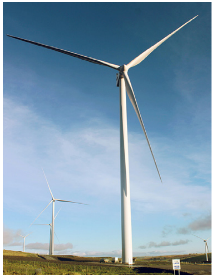
The wind farm will be capable of providing renewable electricity to meet the average needs of more than 26,000 homes.
