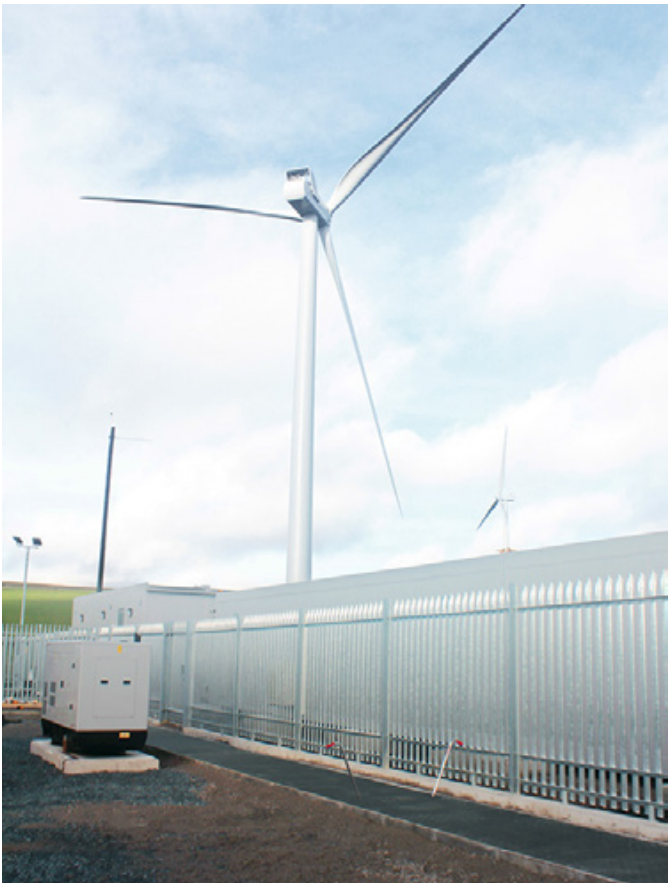
Fibrelite D400 trench covers on wind farm substation
