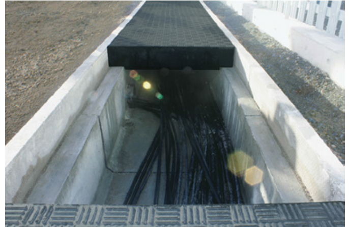
Slit trench with stepped covers over electrical cabling
