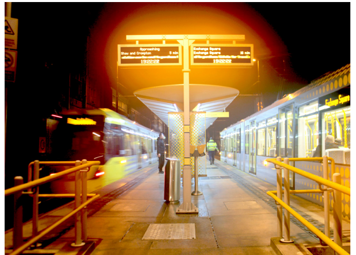
Fibrelite covers provide a safe walking surface in all weather conditions
