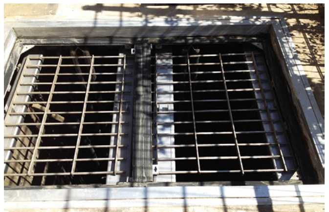
Removable beams hold safety grid
