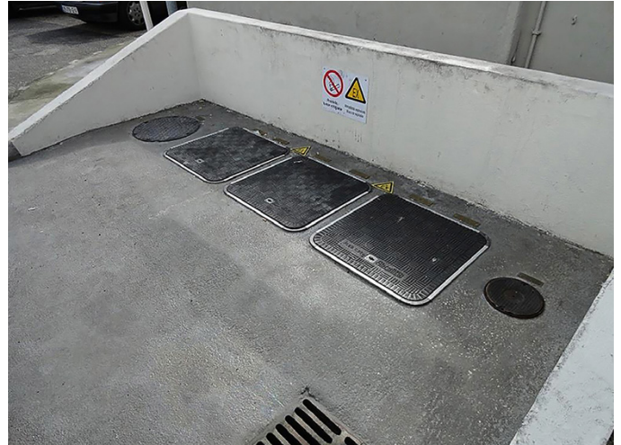
Recently upgraded site with Fibrelite's 600mm sq. 25 tonne load rated covers (FL60)
