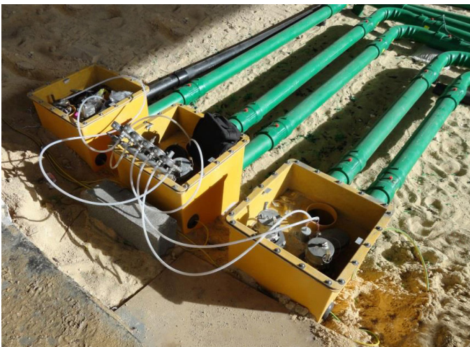
Secondarily contained Fibrelite remote fill sumps
